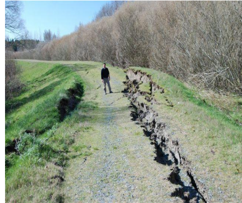
Slumping and lateral spreading observed on stopbanks on Waimakariri River following earthquakes in Sept 2010, Source: Environment Canterbury
